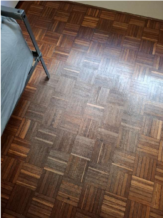
Slight damage on the floor
